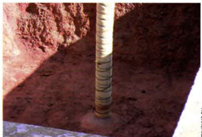
Deep recharge bore well
