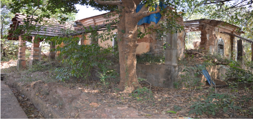
8.6: A dilapidated 'empty' house in all sense in Cuncolim
