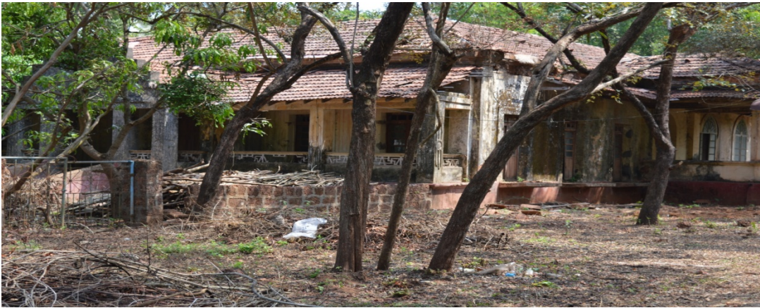
8.7: A dilapidated 'empty' house in all sense in Baga-Velim
