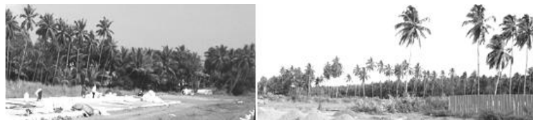
Figure A17.4 TGSB getting cut and damaged by the new Highway construction at Agasaim
