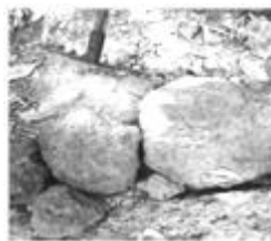
Figure A15.36 Backfill, stabilized with 10% ash and 4% lime then raked to mix in
