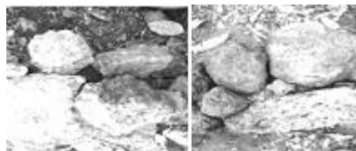
Figure A15.35 Two layers of dry rubble masonry per course and gap filled with smaller stones to pack them.
