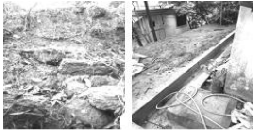
Figure A15.32 Collapsed masonry portion and proximity of completed wall to the Borges house and neighbours' house
