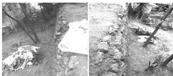
Figure A15.38 Two views of the completed wall built using TGSB technology.
