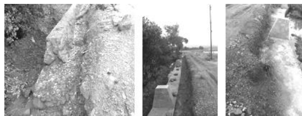
Figure A15.15 Bad embankment repairs-Rubble, PCC and masonry all above the riverbed.
