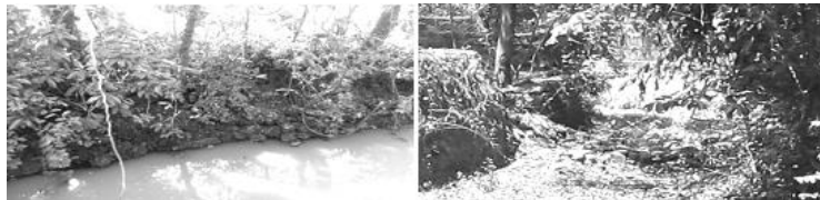
Figure A17.3 Pilferage of facing material and overgrowth of other trees and collapsed new cemented stone masonry wall at Curtorim
