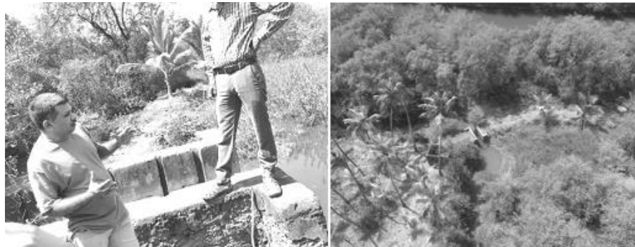
Figure A15.23 Site inspection and aerial view of sluice gate at Kolya Khazan
