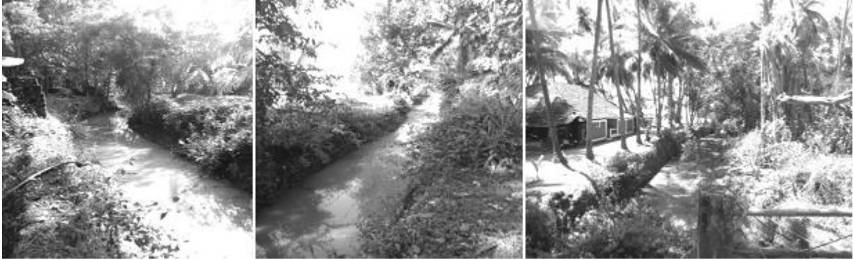
Figure A15.30 The damage to the 3 m bund protecting the wanvodd
