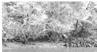
Figure A17.5 Fallen & dead mangrove, damaged & missing pitching, disappeared TGSB and bluish grey marine soil at Diwar
