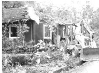
Figure A10.2 Roof of residences damaged by wind. The shovel was used to clear the fallen trees)
