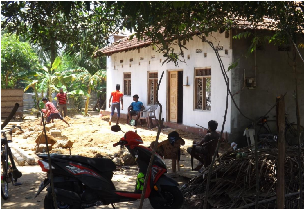
Photo 1: Being an owner-driven model sets the Indian Housing Project apart, since the beneficiary and his friend, family and neighbours participate in the construction process
